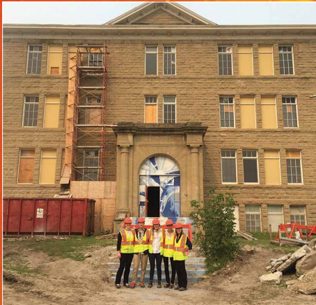
NATIONAL's Calgary team on a hard-hat site tour of the King Edward building, which is being renovated as a creative work space for cSPACE artists. Left to right: Nichole Budd, Howie Thomson, Heather Reinsborough, Mallory McCredie and Caitlin Sparks
